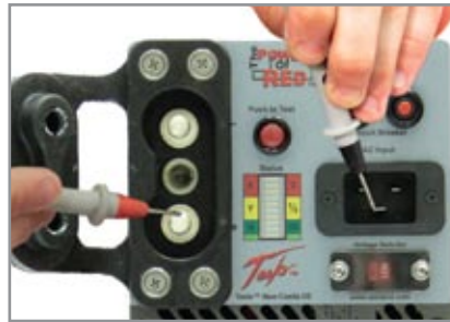
2. Place the negative probe on the ac ground post and the positive probe to the dc positive post. Multimeter should read greater than 10 M \Omega .
