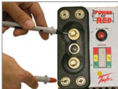
2. Place the positive probe to the fastener screw on the dc receptacle. Move the negative probe to the dc negative post. Multimeter should read 0 Volts.
