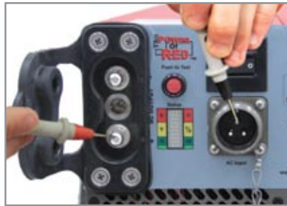
2. Place the negative probe on the ac ground post of the ac input and the positive probe to the dc positive post. Multimeter should read greater than 10\text{ M}\Omega .
