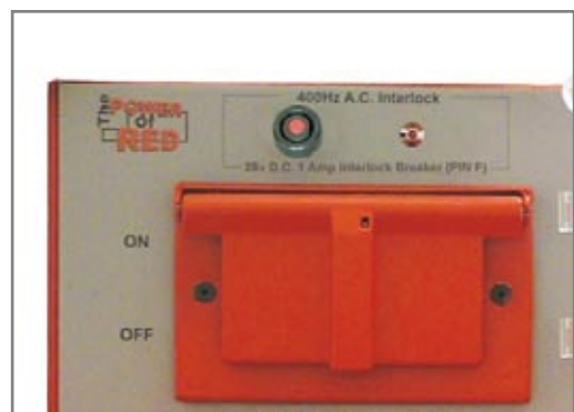
Figure 4.12.2 - 400Hz Interlock Breaker
