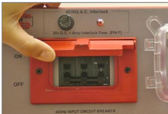
Figure 8.2.15 400Hz AC Input Circuit Breaker (set to “OFF” position)
