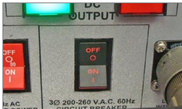
Figure 8.2.16 60Hz AC Input Circuit Breaker (set to “OFF” position)
