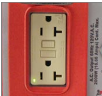
Figure 6.4.4 60Hz 120 Volt AC Outlet with GFCI receptacle.
