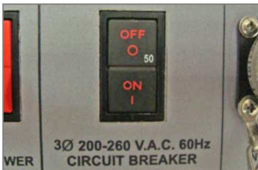
Figure 5.2.3 - 60Hz AC Input Circuit Breaker set to the “ON” position.
