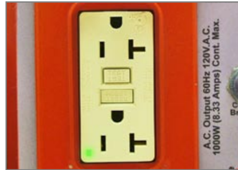
Figure 11.1.7 – 60Hz AC Power Outlet “ON” (green LED illuminated)
