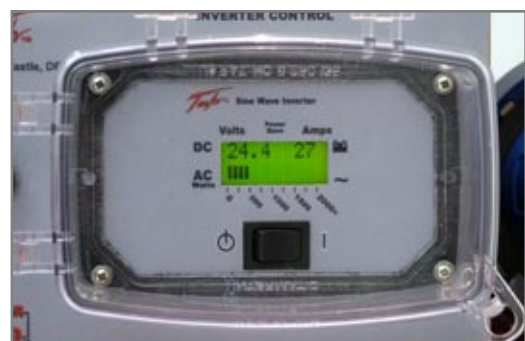
Figure 4.16.2 Inverter Display Panel
