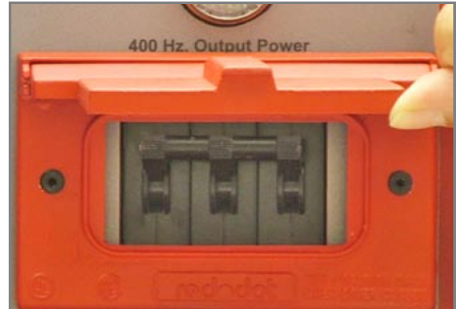
Figure 6.3.2 - 400Hz AC Input Circuit Breaker set to the “OFF” position.
