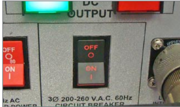
Figure 4.2.2 - 3-phase 60 Hz Input Circuit Breaker
