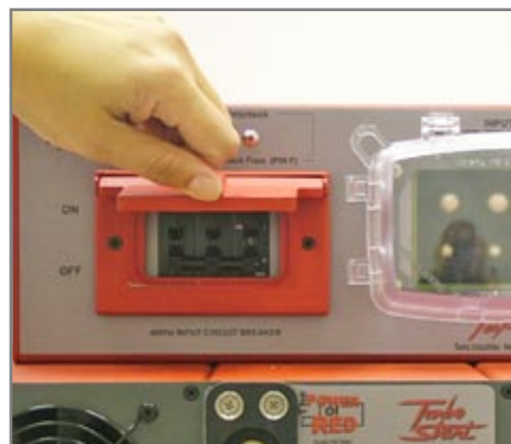
Figure 4.10.2 - 400 Hz AC Input Circuit Breaker
