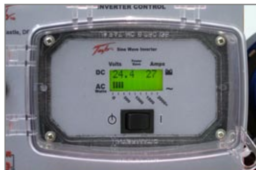
Figure 6.4.2 Inverter Display Panel with Switch set to “I” (ON) position.
