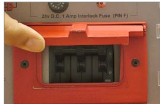
Figure 5.2.4 - 400Hz AC Input Circuit Breaker set to the “ON” position.
