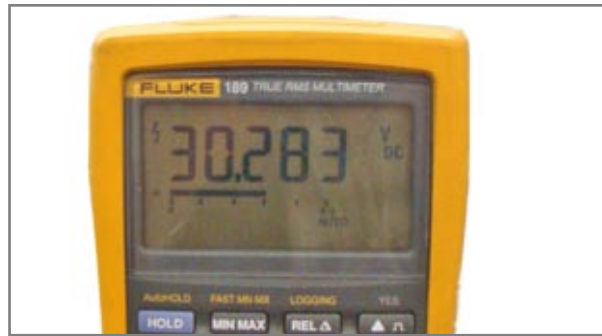
Figure 8.2.17 – Multimeter reading typical power cell voltage (with AC power)
